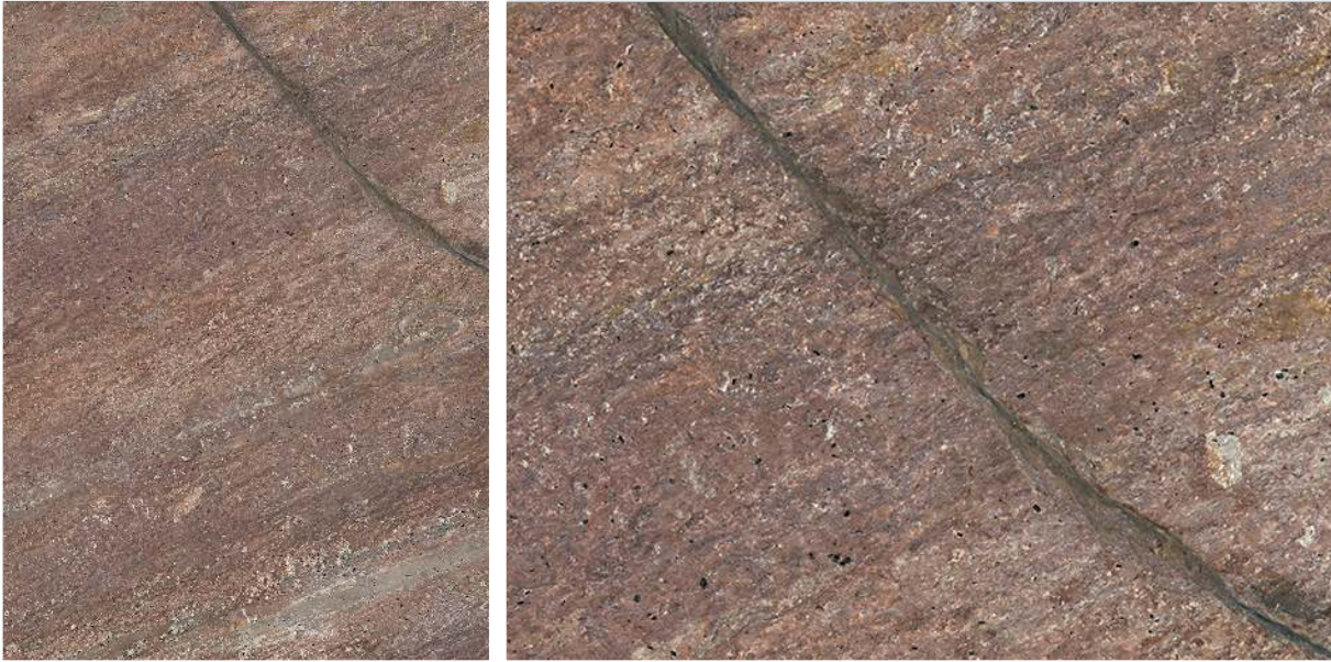
Broken red tile
